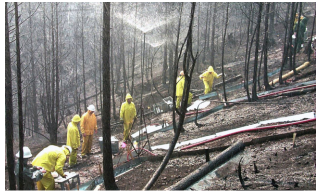
Figure 3. A photograph of the rainfall simulation experiment in progress. Three plots are visible in the photograph: the nearest plot is treated with a contour-felled log, the middle plot is untreated, the far plot is treated with a straw wattle
